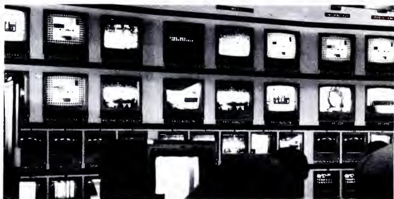
Central control switching room included 48 monitors displaying input and output signals from the venues.
